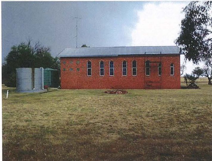
Figure 4 View south from the northern extent of the property to the existing northern facade.
