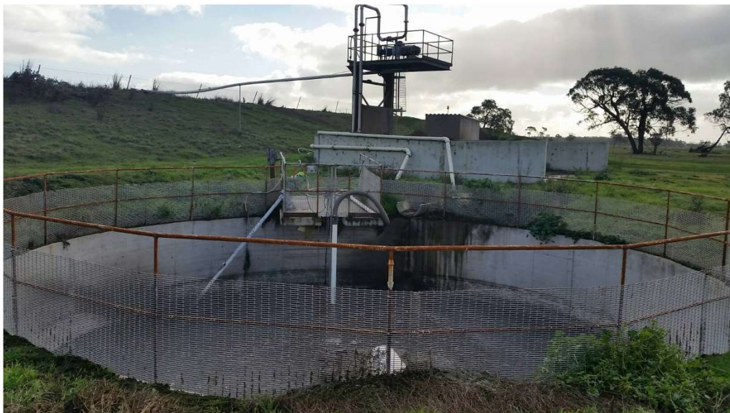
Photograph 3 – Sump and Screw Press Separator
