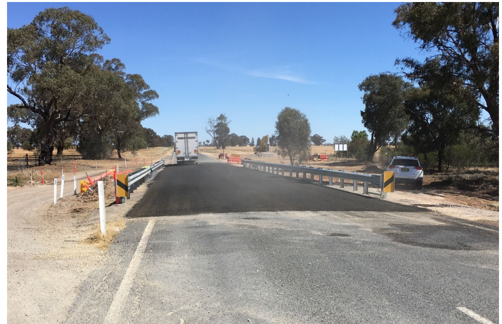
Stage 2 Flood Mitigation Works in Lockhart were completed in the 2019-20 year, including an upgrade of the major culvert on Albury Road.
