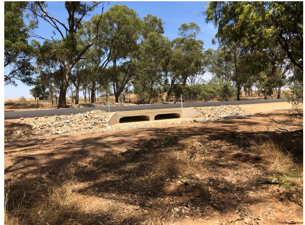
The Heavy Vehicle Safety & Productivity Program grants allowed Council to upgrade major culverts, including this one on Lockhart The Rock Road, across the Shire to enable higher mass limit access on Council's road network.
