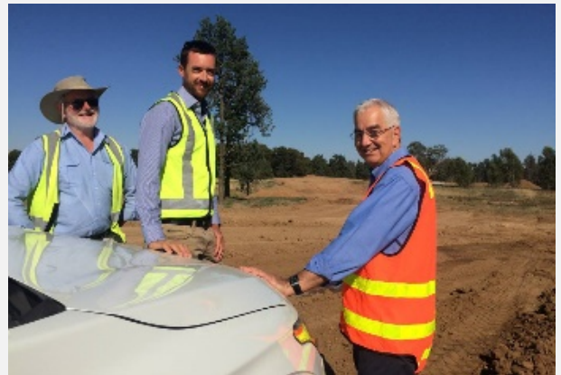
Former Project Officer, John Geppert, former Manager Environmental Services, Alan Gundrill and General Manager, Peter Veneris, inspecting the flood mitigation works at Lockhart.
