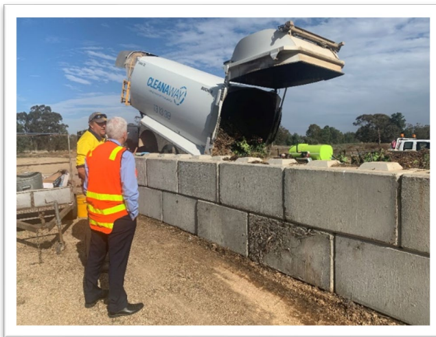
Council’s General Manager, Peter Veneris, and Waste Supervisor Ed Schneider, inspect the new FOGO (Food Organics Garden Organics) processing area at the Lockhart Waste Facility.
