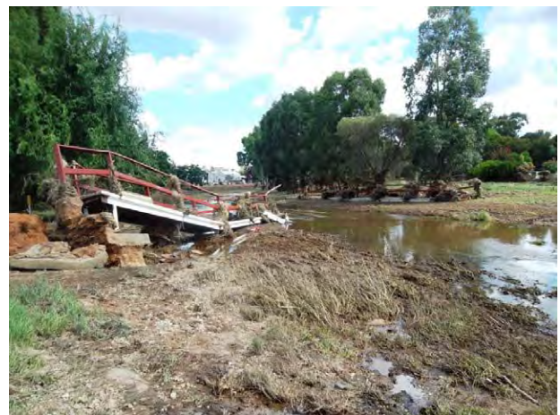
Image 3: Destroyed footbridge at Green Street (source: Reference 3)
